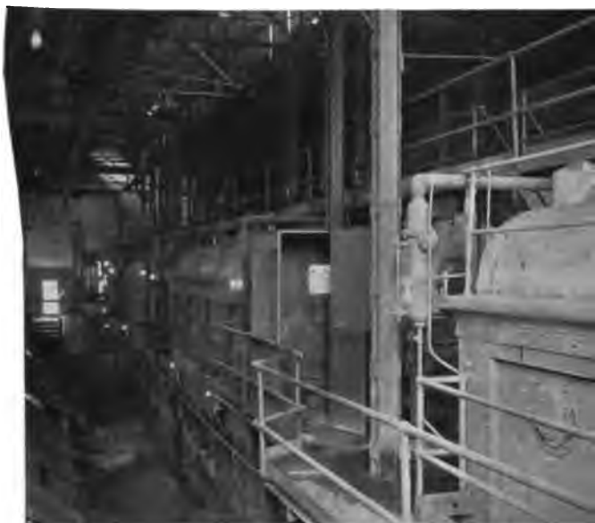
Fig. 1. Foot-walks and Runways in Boiler Plant.*
